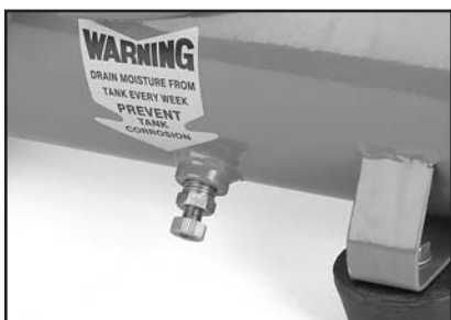
Figure 10. Tank drain valve.
