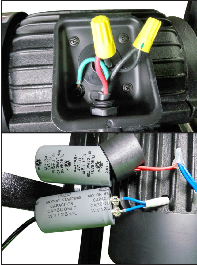
Figure 61. G1066Z drum motor connections and capacitors.
