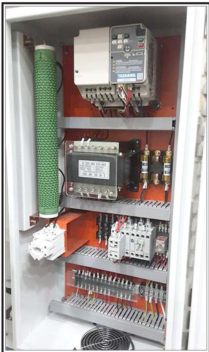
Figure 67. Electrical panel wiring.
